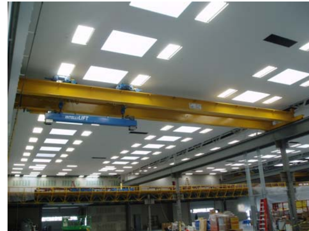
Figure 1 – IntelliLift on Crane
