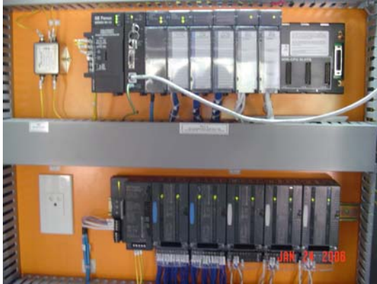
Figure 3-General Electric Rx3i Programmable Logic Controller used for the Stands, Shears and Pinch Rolls with Ethernet Communication to the drives.
