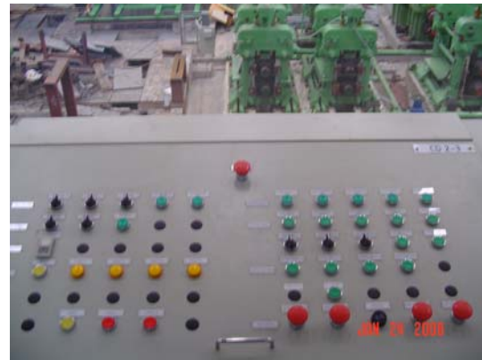
Figure 5-Operator Control Desk in Main Pulpit
