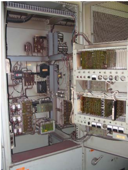
Figure 2 - Existing Westinghouse Regulator
