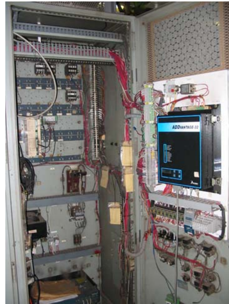
Figure 3 – Avtron Retrofitted Regulator
